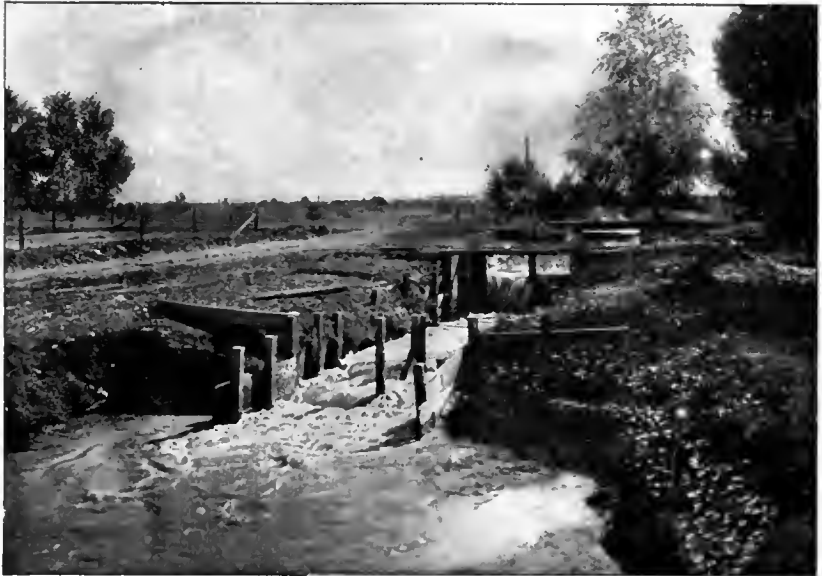
No. 2—Main Check, Redwood Canal, Near Holtville, Imperial County, California. Courtesy Henry R. Worthington Hydraulic Works, New York.
