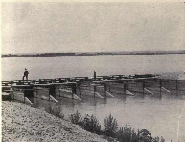
B. HEAD GATES OF FARMERS AND MERCHANTS IRRIGATION COMPANY ON PLATTE RIVER, NEAR COZAD, NEBRASKA.
