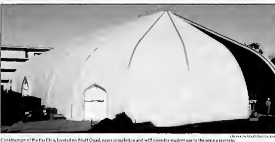
Construction of the Pavilion, located on Bruff Quad, near completion and will open for student use in the spring semester.
