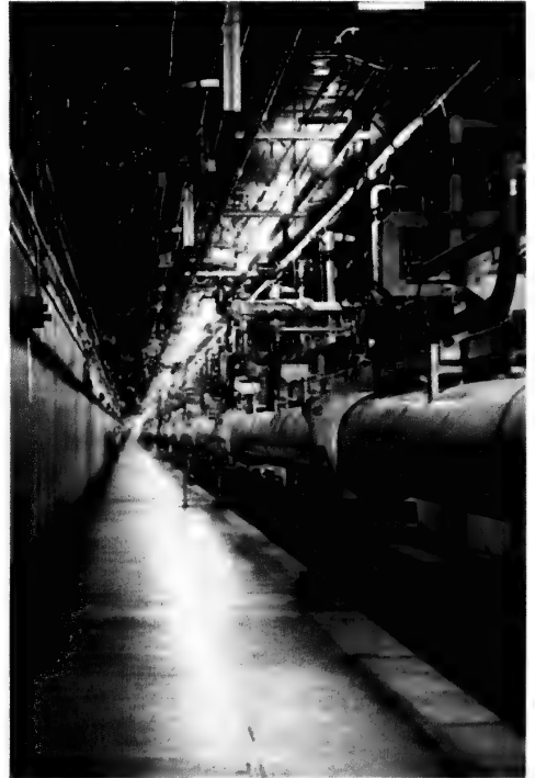
Figure 4: A view inside the two-mile SLAC accelerator tunnel showing the linac mounted above the alignment light pipe.
