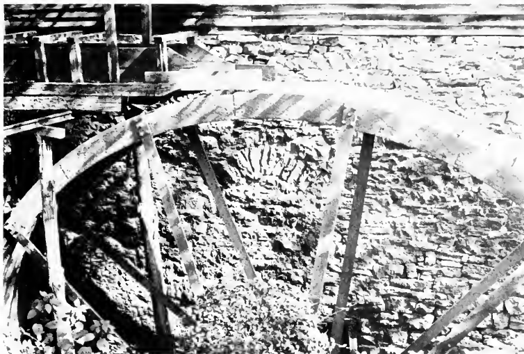
Figure 2. Detail of a portion of the limestone foundation of Zane's grist mill on Cedar Creek; the wheel and structure above are twentieth-century.
