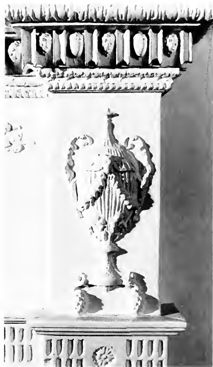
28b. Truss block of a mantel with composition ornament by the firm of Zane, Chapman, and Wellford. John Steele House, Salisbury, North Carolina. HOA 8 \frac{1}{8} " , WOA 4". MRF 27,287. The pineapple and acorn, beading, and tongue decoration, all composition ornament specified in Zane and Chapman's bill to Steele, are effectively combined with the punch-and-gouge work of this mantel.
