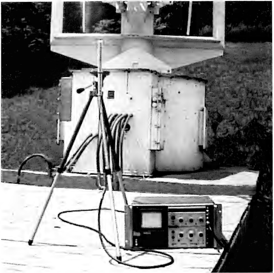
Figure 6. Morehead Radio Telescope, Morehead State University, Morehead, Kentucky. The dipole antenna and spectrum analyzer receiver system are shown.
