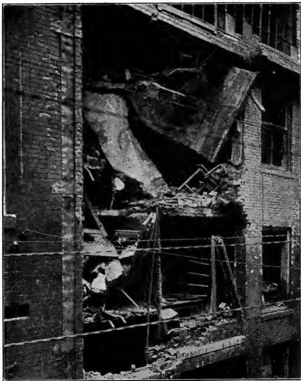
FIG. 3. A Pittsburgh film exchange fire; exchange not sprinklered. Showing wreckage due to explosion, and spalled brickwork from intense heat when gases of decomposition reached outside air where there was sufficient oxygen to completely burn.
