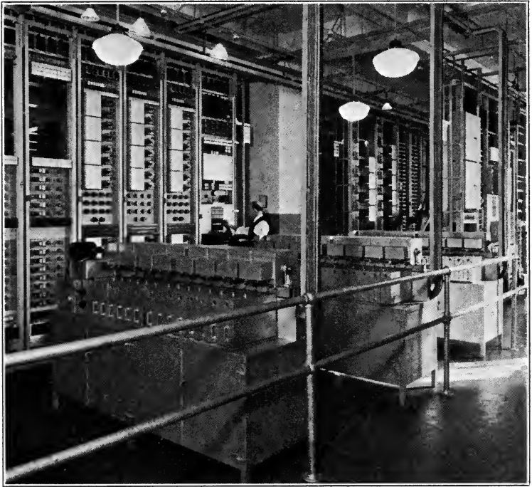
FIG. 2. Commercial installation of call-announcing apparatus. At the left can be seen the frames carrying the telephone repeaters which form the last stage of amplification, together with other telephone apparatus.
