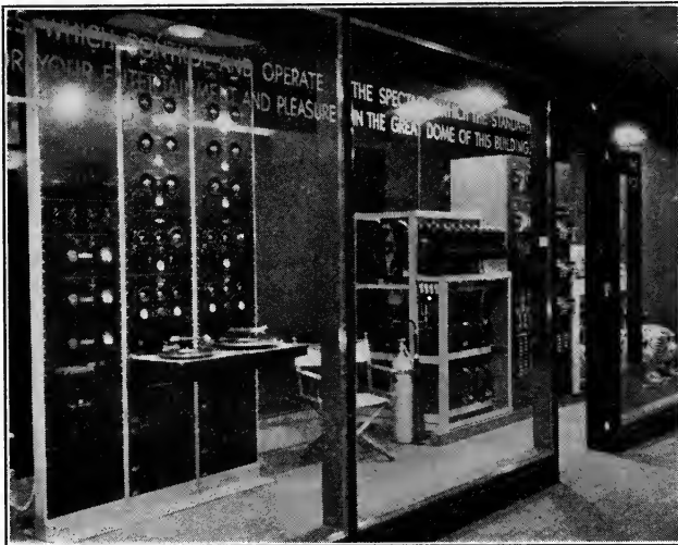
FIG. 5. Standard Oil Co. of Indiana control room.
