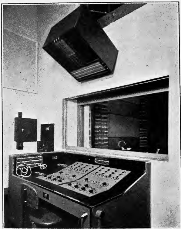
FIG. 2. View of re-recording console, showing double glass window, which may be opened into stage D . At the top may be seen the compound baffle used for monitoring, and the window through which pictures may be projected upon the screen in stage D from the projection room (on the upper floor at the right, not shown in the picture).
