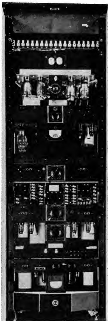
FIG. 5. Program rack with front cover removed.
