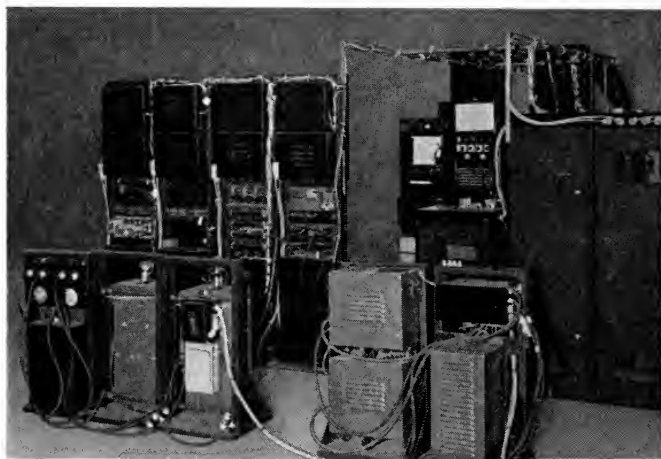
FIG. 8. Power equipment. In the foreground are rectifiers to supply low voltage direct current to loud speaker fields and exciting lamps in the machines. The next row consists of power amplifiers ( left ) and plate and heater-supply equipment in the three cabinets at the right.
