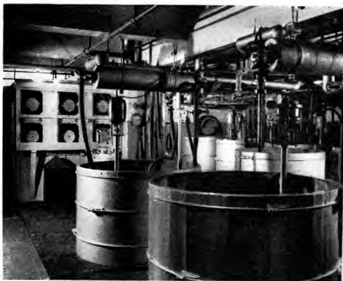
FIG. 4 General view of Chemical Department installation.
