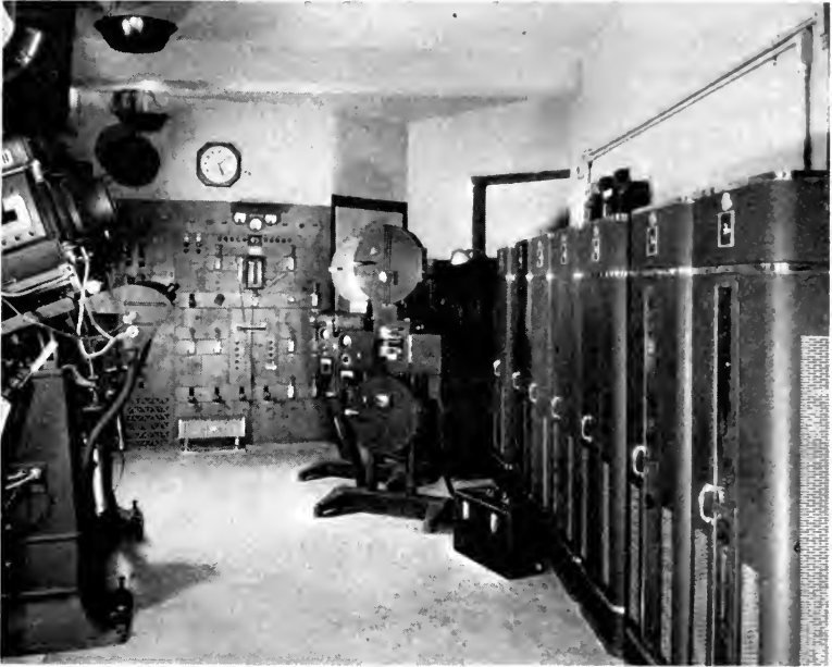
FIG. 2. Installation in the Carthay Circle Theater, Hollywood.
