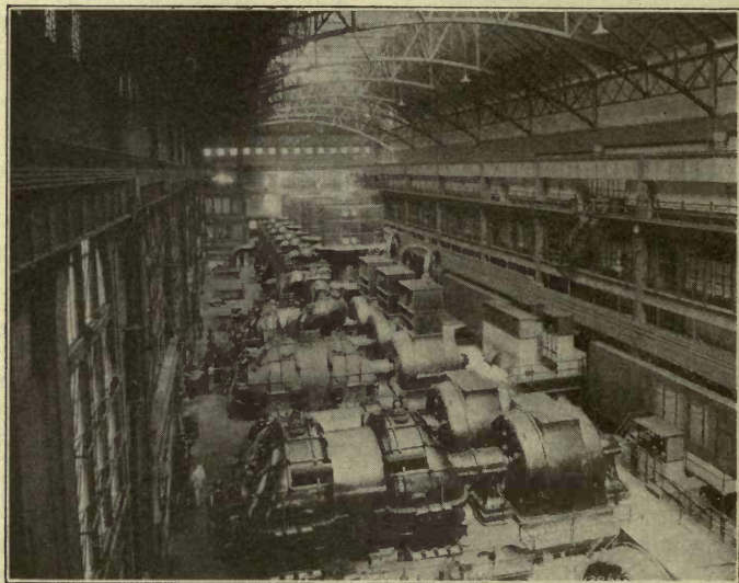
Fig. 141. — Westinghouse electric generators in the 74th Street Station of the Interborough Rapid Transit Co., New York City.
