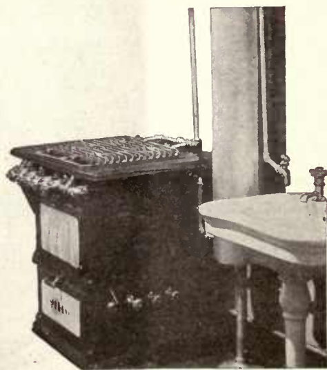
The hot water grate in place.
