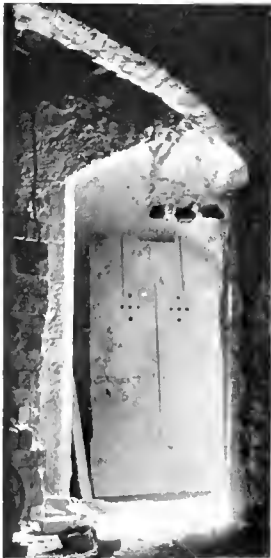
Fig. 13. The dividing transverse wall adapted to an earlier existing doorway by an arch.
