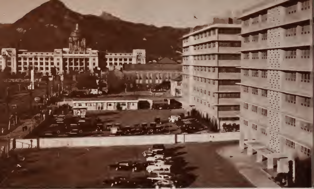
Newly-built office for the Supreme Council for National Reconstruction (center) and the war-damaged Capitol Building under repair, Seoul.
