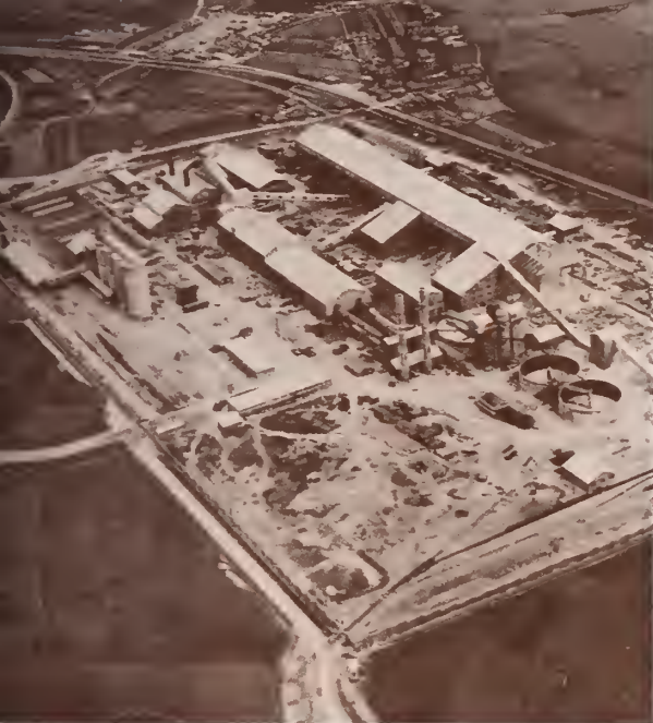
THE GIANT NEW MUNGYONG CEMENT PLANT , built with U. N. aid, is a hive of activity among the rice paddies of a Korean valley.
