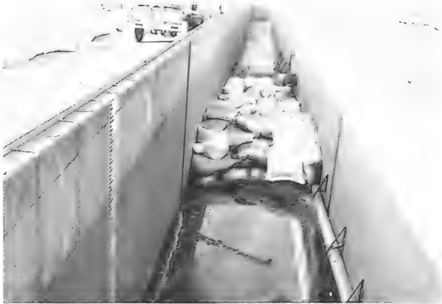
Figure 29. Repairs to structure II and first layer of bags for structure III (test III).
