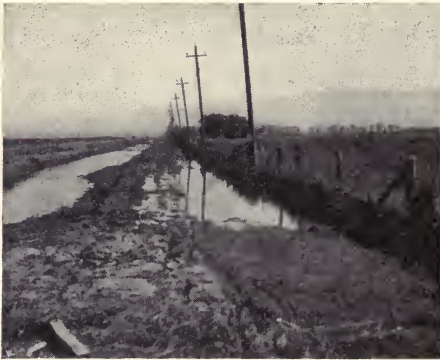
FIG. 89. A road badly in need of drainage.
