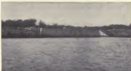
FIG. 75. A large concrete tide box at Clatskane, Oregon. There are five outlets each five by six feet.
