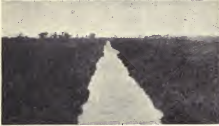
FIG. 57. Drainage outlet canal from Devil's Slough drainage district, Illinois. Represents a canal in good condition.
