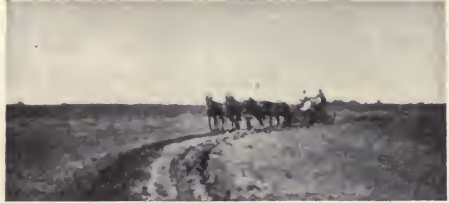
FIG. 35. Filling the tile trench with a road grader. (Courtesy Iowa State College.)
