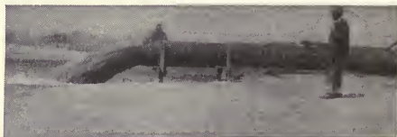
FIG. 65. The discharge pipe of the dredge shown in Fig. 64.
