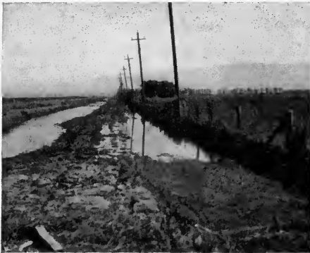
FIG. 89. A road badly in need of drainage.
