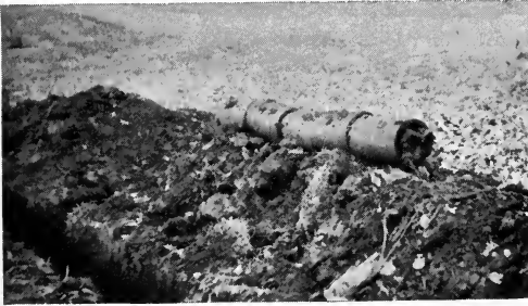
FIG. 82. Tile drain filled with silt due to poor outlet.
