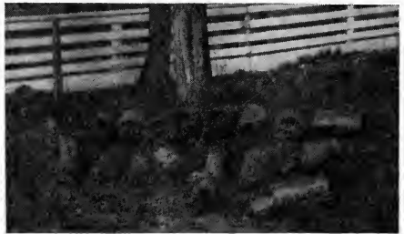
FIG. 40. Drain filled with roots from adjoining willows. (Courtesy Iowa State College.)
