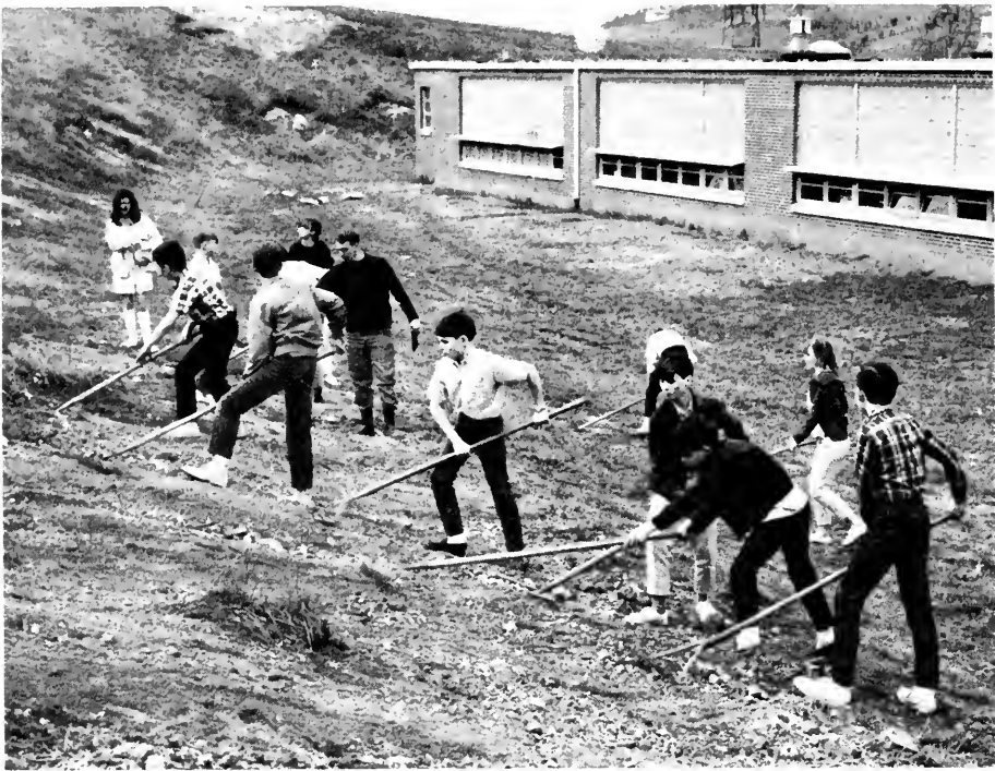
Learning to control soil erosion on a Tennessee school site means shaping and seeding the slope to appropriate grass seed mixtures to protect the soil from water runoff.
