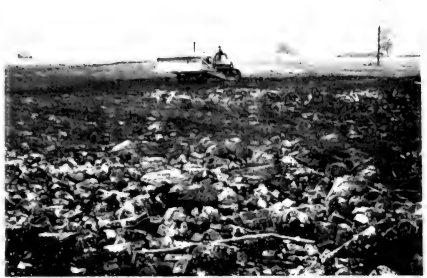
Fig 6.2 Bulldozer spreading thin layer of coke breeze over consolidated brick tunnels. Foreground shows sections of tunnel still requiring to be broken and covered.
