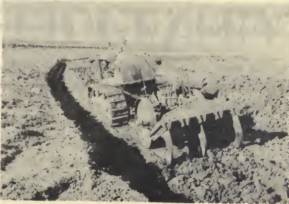
Ripper loosening compacted soil in terrace channel. Earth will be removed with a rotary fresno to build up a low place in the terrace ridge.
