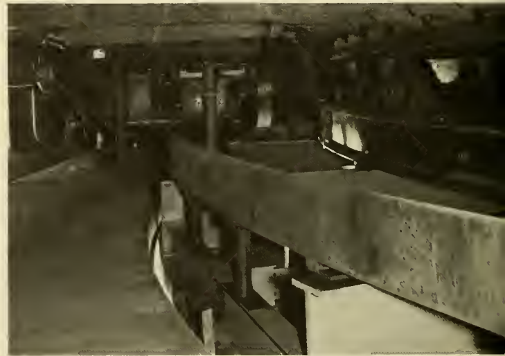
One of two motors used to change a chapel into an auditorium.
