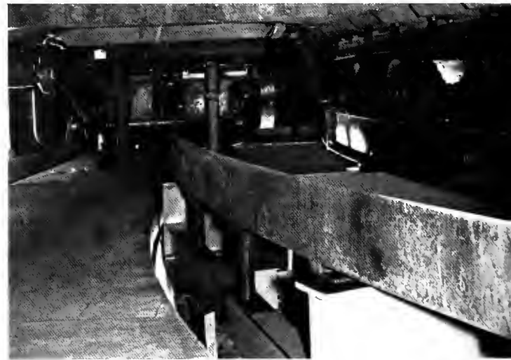
One of two motors used to change a chapel into an auditorium.
