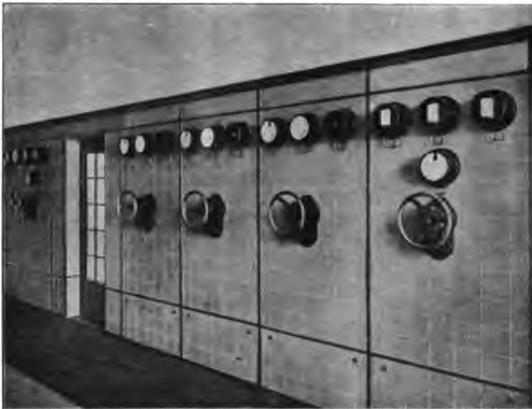
Fig. 83.—Operating Gear for Feeder Oil Switches.
