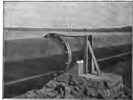
Fig. 155.—Compressed Air Plant. 24-in. Pipe ; method of fixing the Pipe above ground on a straight section.
