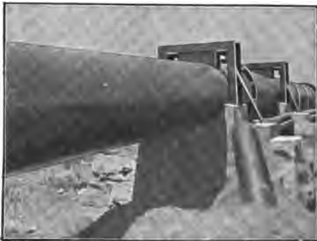
Fig. 156.—Compressed Air Plant. Method of fixing the Pipes above the ground. Fixed point.
