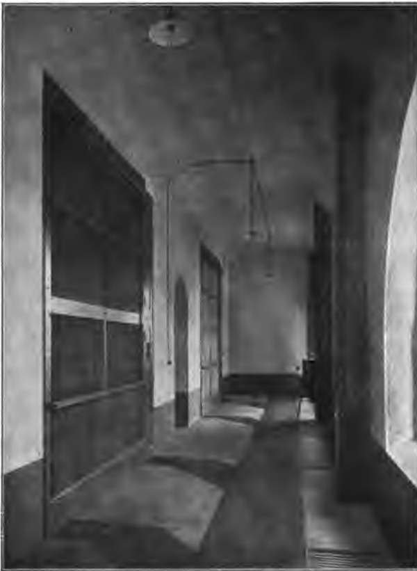
Fig. 78.—Air Filter Passage in the Engine Room Basement.
