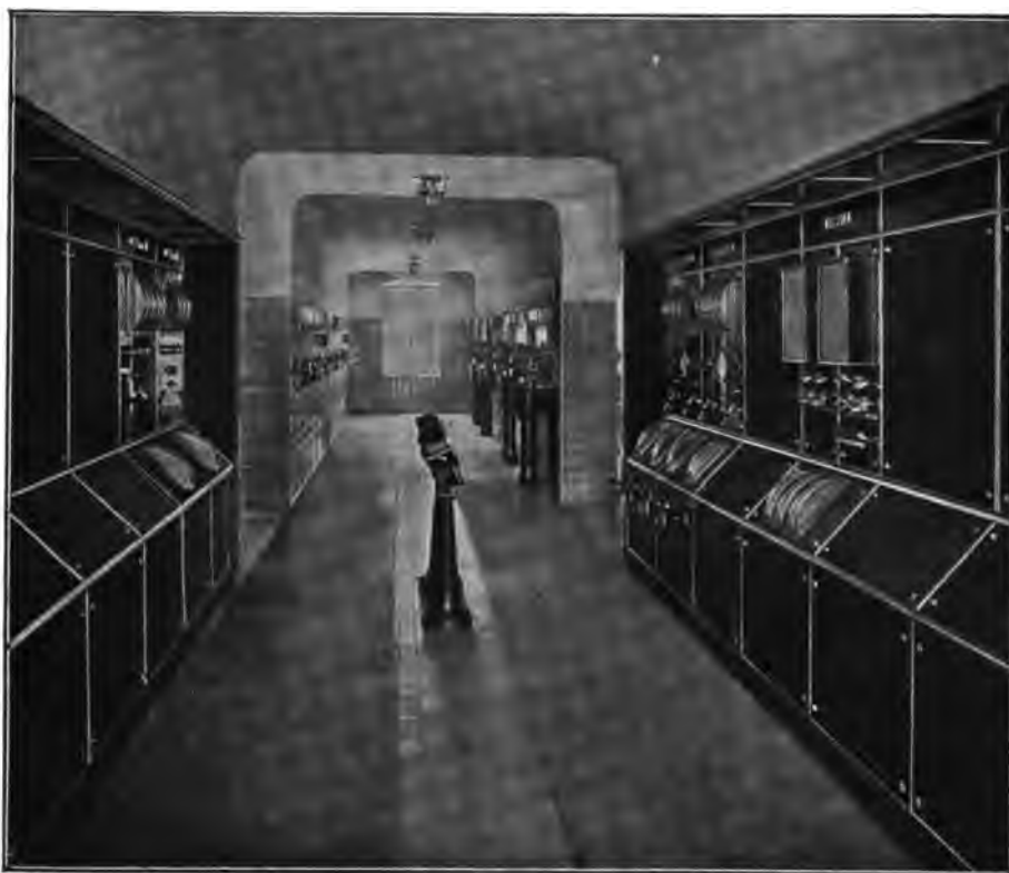
Fig. 85.—Control Passage in Switch House.
