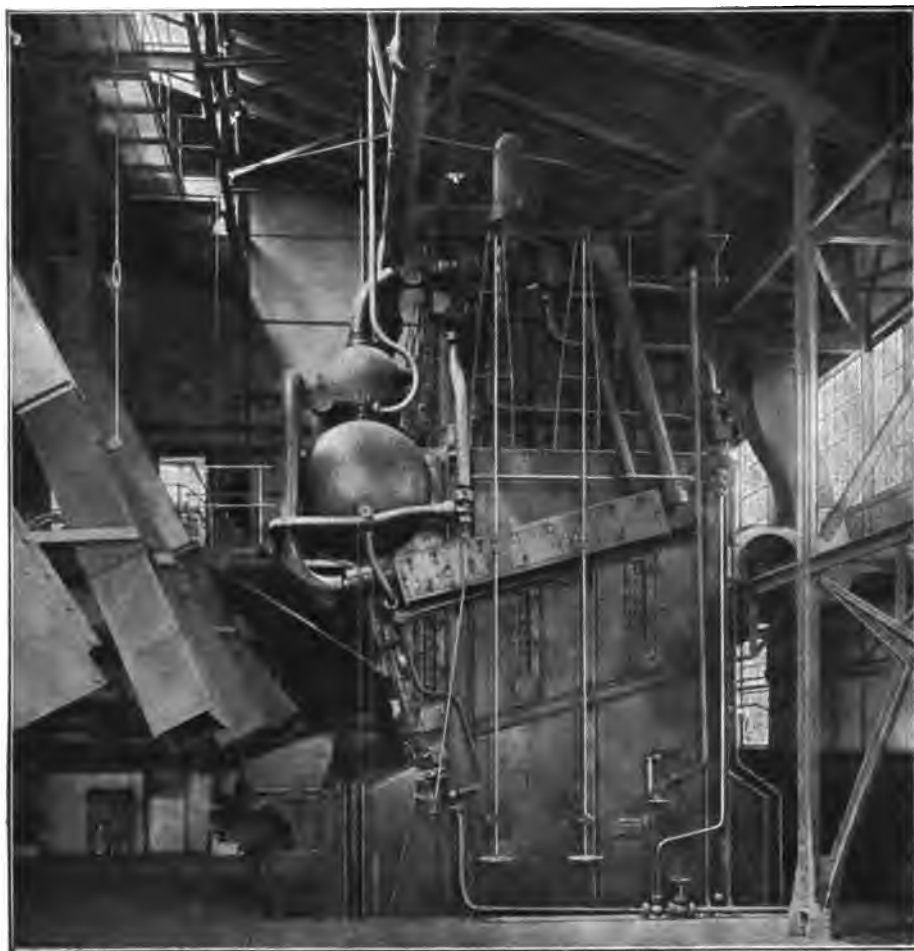
Fig. 71.—End View of One Boiler Unit.
