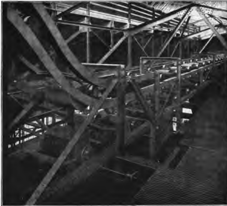
Fig. 68.—View of Coal Conveyer in the Roof of Boiler House. Scale, 1 to 200.
