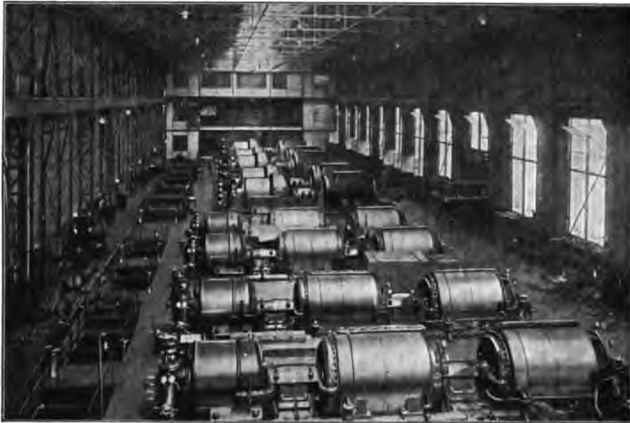
Fig. 137.—Rosherville Power Station. View of the first Lay-out complete : 5 Generators, 4 Compressors.
