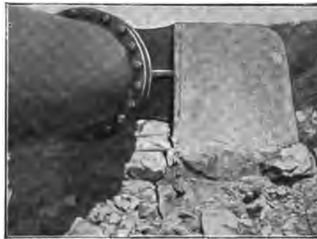
Fig. 157.—Compressed Air Plant. Anchor for a 30-in. bend above ground. The illustration shows how the pillar has given way owing to the inadequate foundation.
