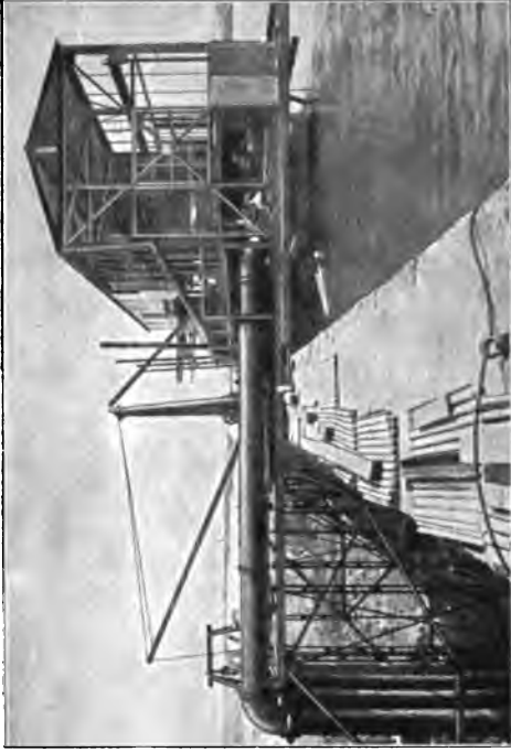
Fig. 131.—Rosherville Power Station Pumping Plant. Pump House in course of erection, with a portion of the Delivery Pipes in position. In erecting the plant the Dam was not made use of at any point, thus complying with the stipulation made by the Mining Companies.
