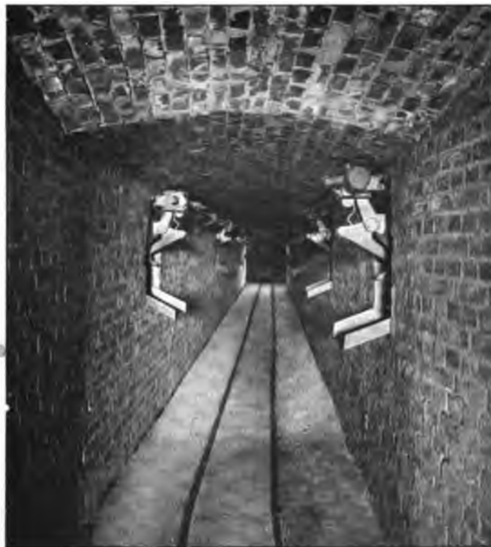
Fig. 23.—Ash Tunnel under the Boilers in the Hirschfelde Electricity Works.
