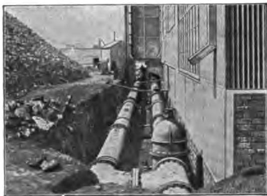
Fig. 149.—Robinson Central Station. Double Pipe Mains for Compressors outside the Building. Centralised Filter Plant for all Compressors visible in the Centre.
