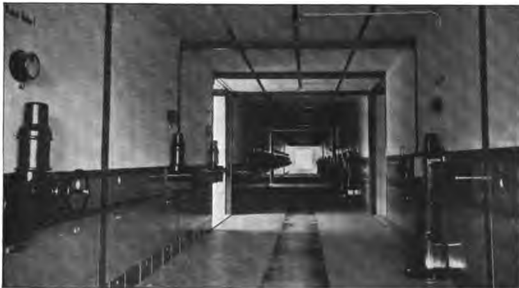
Fig. 26.—Operating Passage for the Oil Switches in the Rheinfelden Electricity Works. In the floor to the right and left are cover trenches for the control wires; the bottom part of panels consists of removable metal plates covering the terminals for the apparatus leads; it is not necessary to enter the high-tension chambers to inspect these leads.
