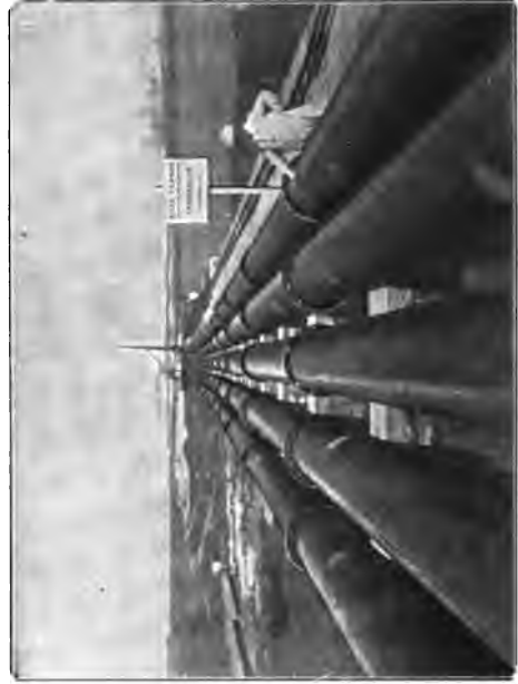
Fig. 132.—Rosherville Power Station Pumping Plant. Laying of the five Delivery Pipes, 25 in. in diameter, from the Pumping Plant to the Inlet Channel.
