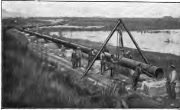
Fig. 154.—Compressed Air Plant. Laying 24-in. Pipe above ground on Masonry Pillars (marshy ground).
