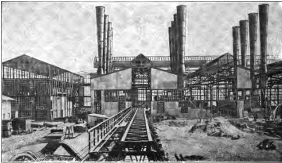
Fig. 125.—Rosherville Power Station. View of the first Coal Conveyor Track, Boiler House, and Switch House. The latter is partially covered with corrugated iron; the first part of the Boiler Plant in the background is in course of erection.
