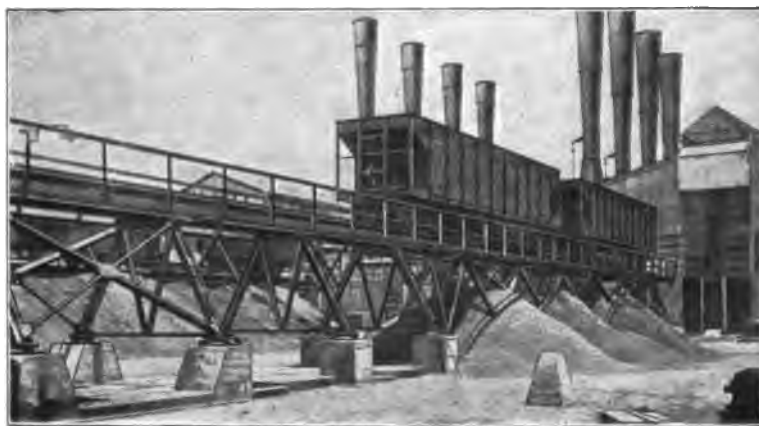
Fig. 126.—Rosherville Power Station. Coal Conveyor Track and two Railway Trucks for Automatic Discharge. Coal Yard underneath and Hoppers for the Bucket Conveyor.
