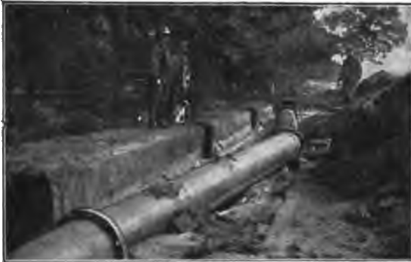
Fig. 158.—Compressed Air Plant. 22-in. Pipe washed out of the Trench as the result of heavy rains.
