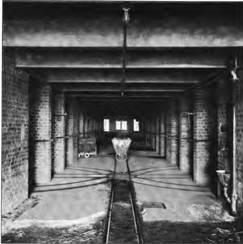
Fig. 21.—Arrangements for the Removal of Ashes in the Basement of the Hirschfelde Electricity Works.
