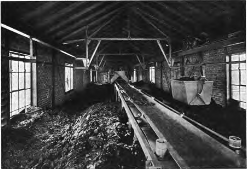
Fig. 18. —Coal Bunker. Ropeway and belt conveyor to carry the coal to bunker.
