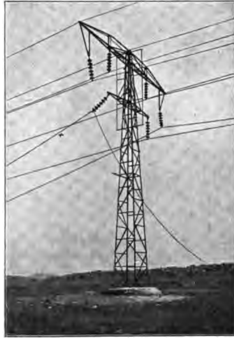
Fig. 177.—Vereeniging Power Station. Experiments carried out on an 80,000-volt intermediate mast in order to find out how the masts withstand breakage of a conductor in the neighbourhood of an anchor mast. The cross shows the length which the conductor has slipped through the suspension clip.
