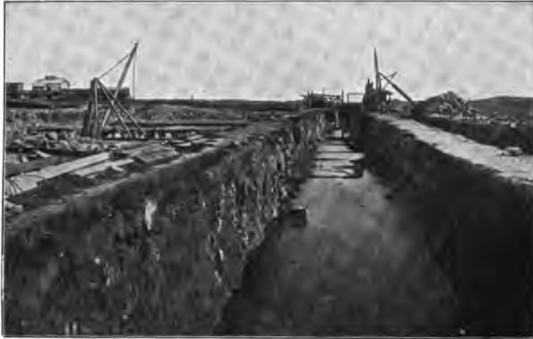
Fig. 133.—Rosherville Power Station. Excavating the Inlet Channel ; Sandy Upper Soil with a Substratum of Rock.
