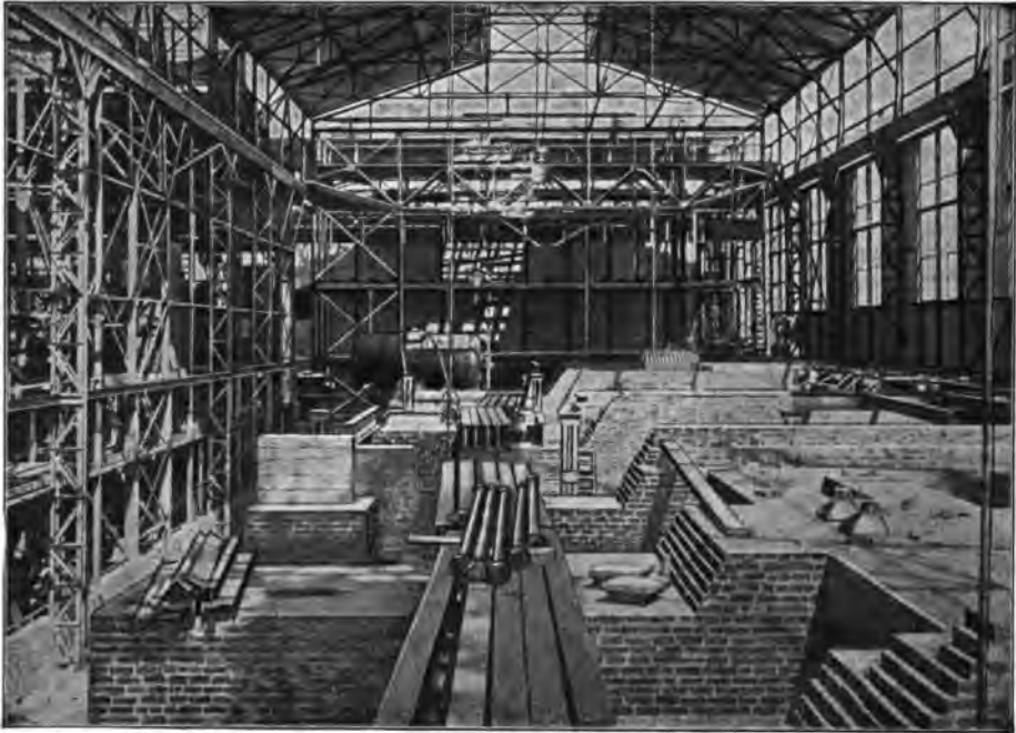
Fig. 135.—Rosherville Power Station. Engine Room with Travelling Crane. Preliminary Work for the Erection of Turbines.
