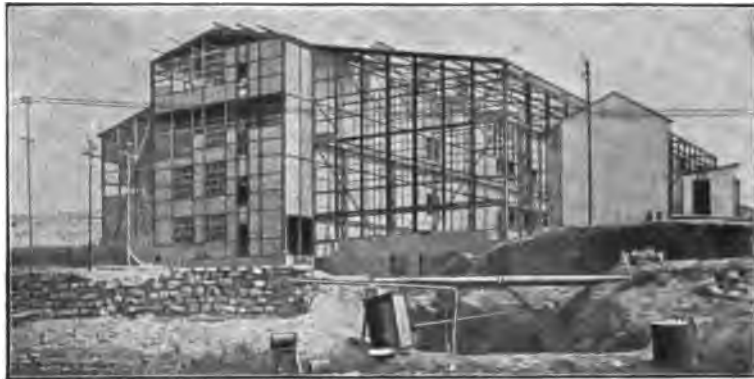
Fig. 146.—Robinson Central Station. Engine Room. Iron Framework completed ready for covering in; on the left, Transformer Cells half finished.
