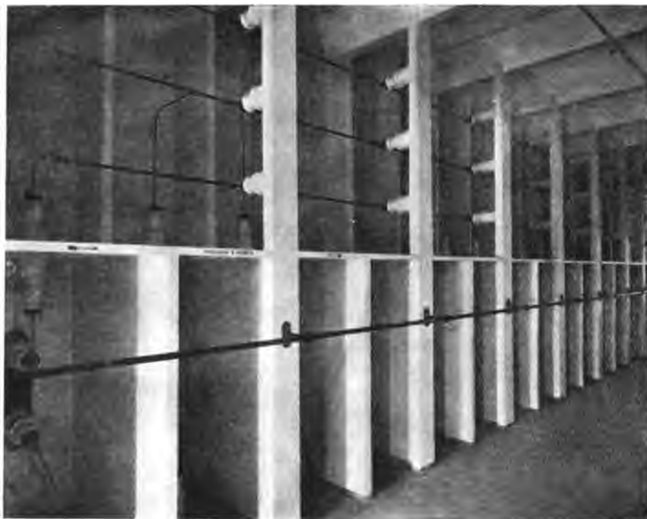
Fig. 25.—Bus-bars in the Hirschfelde Electricity Works. 40,000 Volts. Partitions of Duro Plates. No Partitions between Bus-bars.
