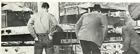
It was a little over a year ago that Blythe Hall looked like this. Inch by inch, the building was lifted hydraulically off the ground.
