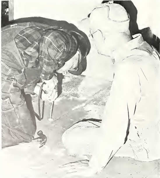
While installing new doors to the Publicotion's Conference Room, the workmen became the subject of another photo.
