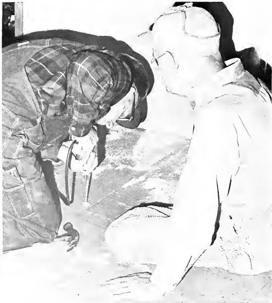
While installing new doors to the Publication's Conference Room, the workmen become the subject of another photo.
