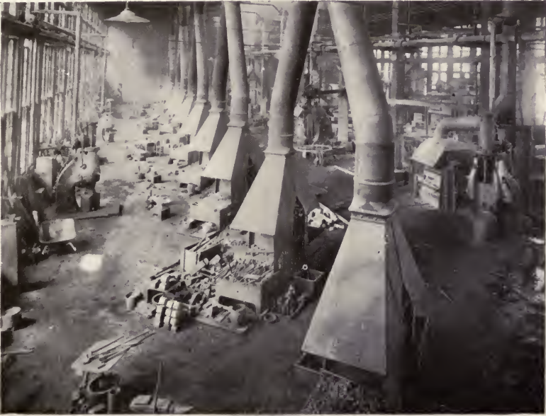
LIGHT AND VENTILATION IN BLACKSMITH SHOP
