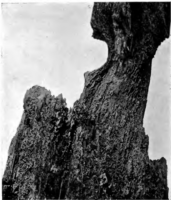
PIECE OF TIMBER FROM RYDE PIER SHOWING DAMAGE CAUSED BY Limnoria AND Chelura (From Brit. Mus. Guide)
