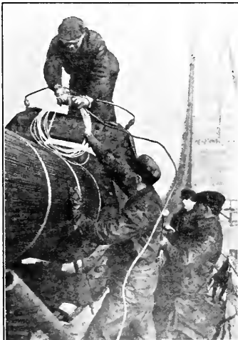
Workmen high up on the Delaware bridge, squeezing cable preparatory to wrapping with wire.
