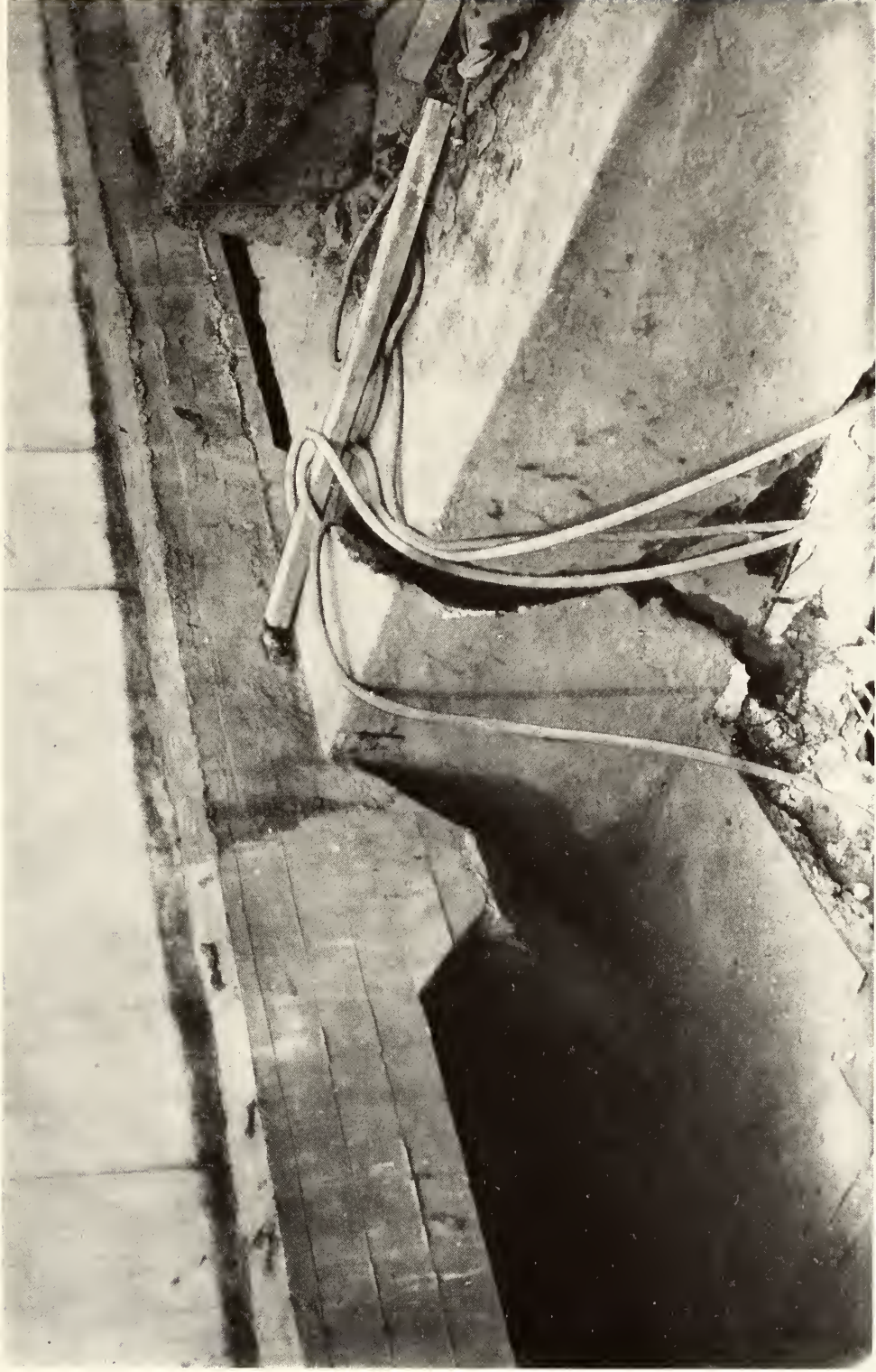
Reinforced concrete slab which originally supported the earthen terrace next to the Memorial, showing damage by settlement before its foundation was carried to bedrock
