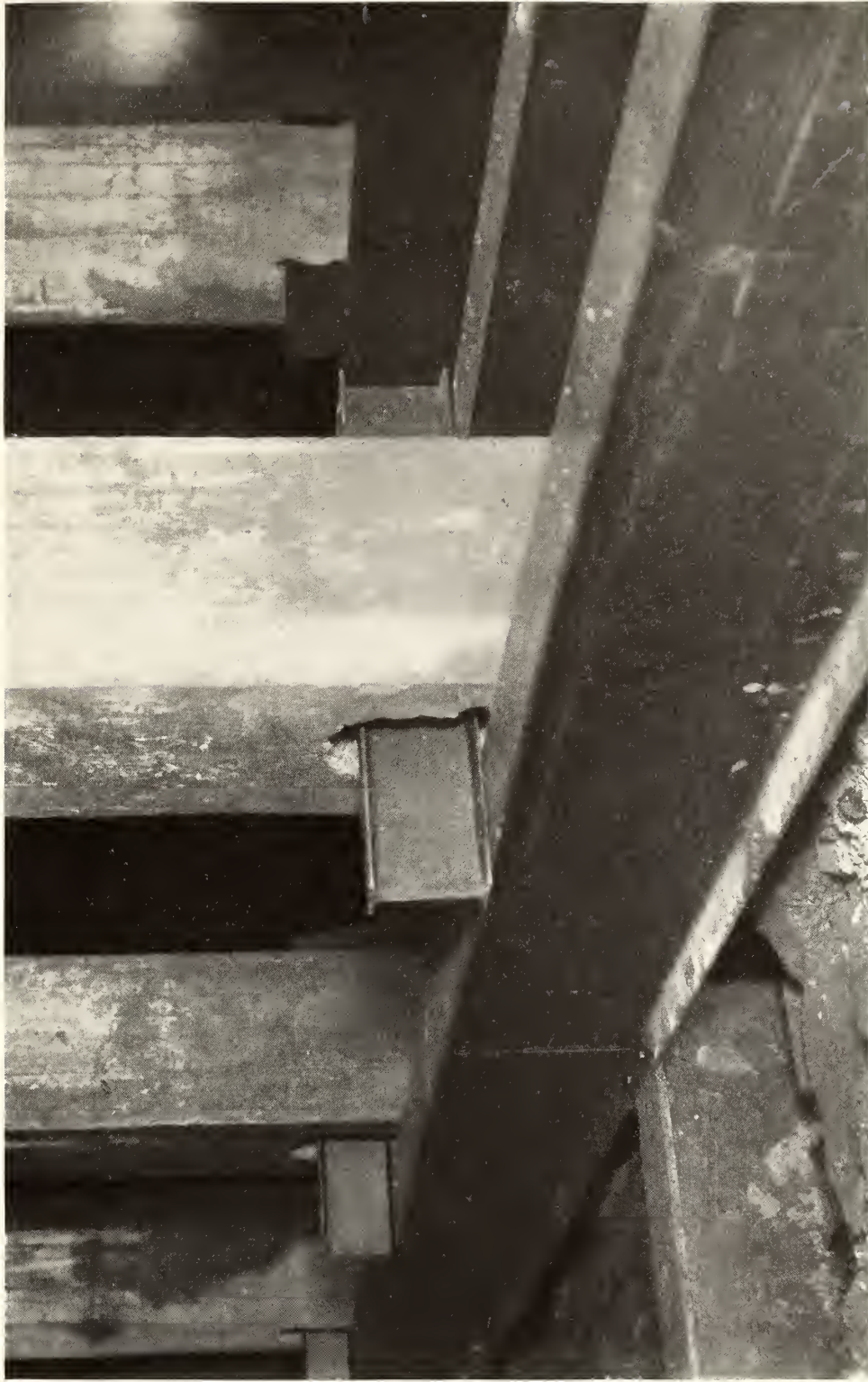
System of steel girders used to support the approaches to the Lincoln Memorial when their foundations were strengthened
