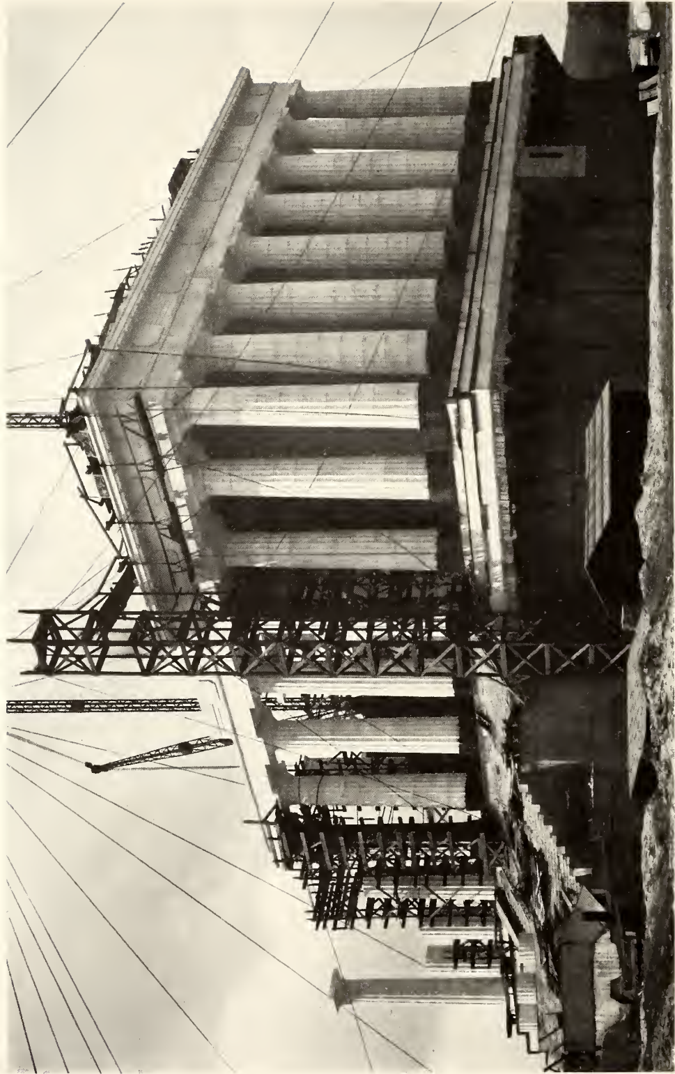
A section of the upper foundation which supports the Memorial, east and north fronts. (About May, 1916)
