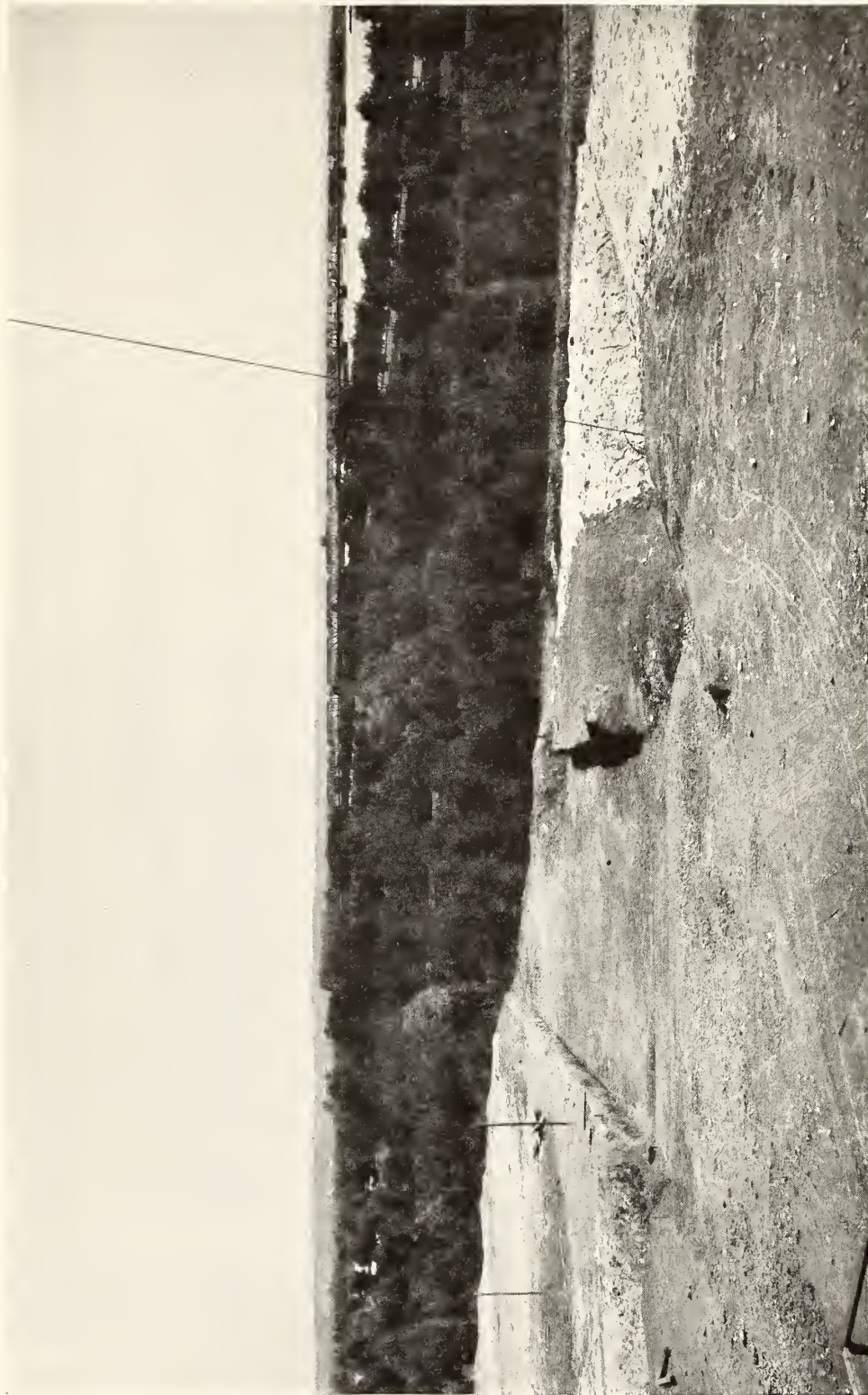
The filling for the earth mound around the Memorial. View looking southwest
