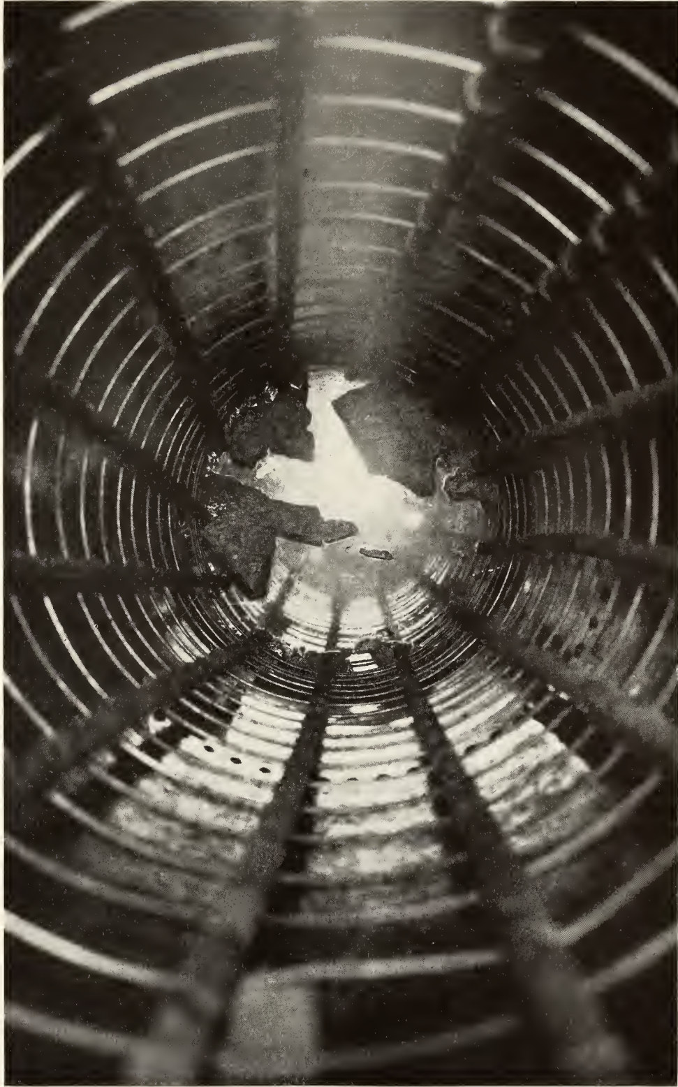
Looking down one of the cylinders used for constructing concrete subfoundation to bedrock, showing reinforcing steel rods. (October 1, 1914)
