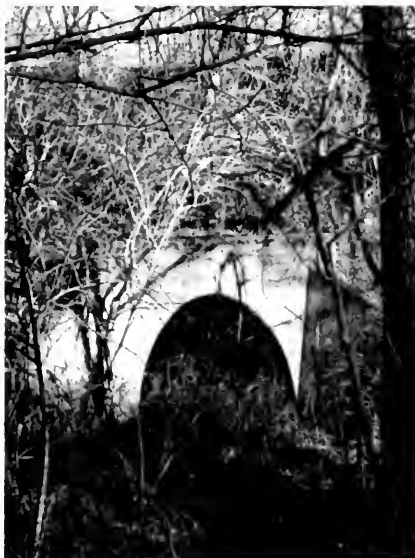
This concrete culvert remains on the north side of Littleton, carrying the MI&L right-of-way over Sugar Creek. Frank Hicks photographs.
