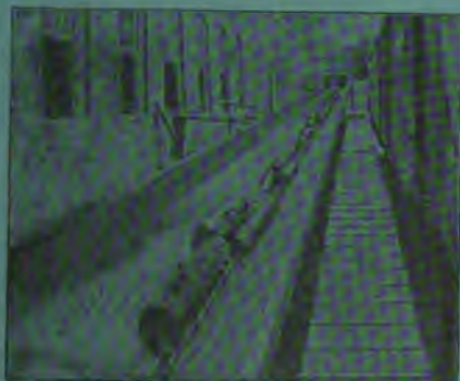
ROLLER CHAIN CONVEYOR
