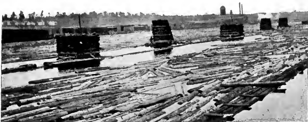
FIG. 108. — Piers built in a River to hold Storage Booms in Place. Minnesota.
