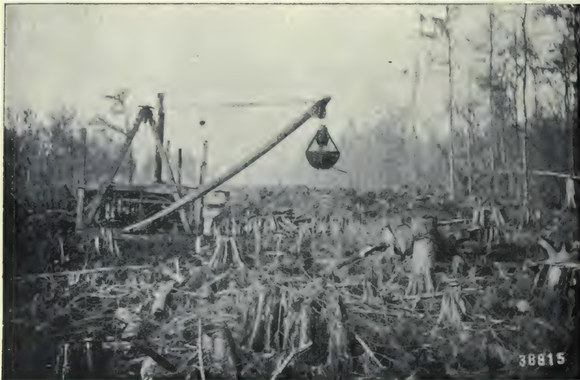
(1). Dredging Canal in Cypress Swamp, Terre Bonne, Louisiana. (U. S. Forest Service Photo.)
