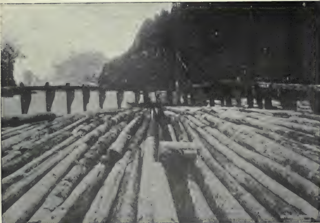
(2). Benson Raft under construction, showing upper part of cradle. Photo by Gifford and Prentiss, Portland, Oregon.
