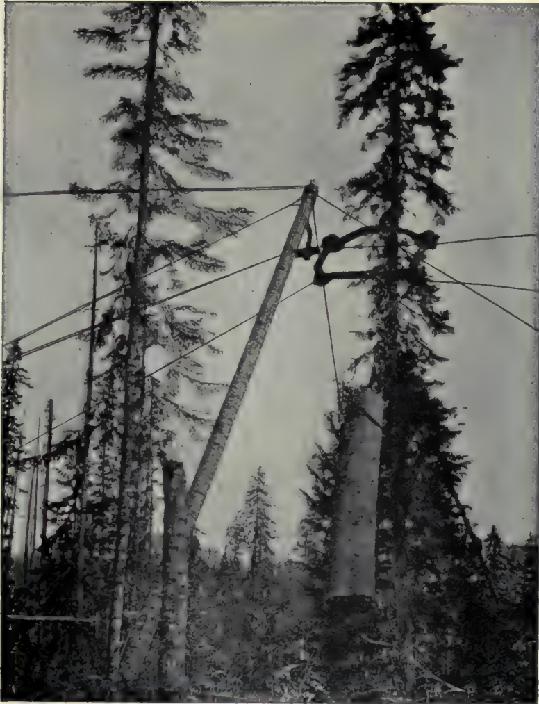
(1). Intermediate support of 3,500 feet overhead rig ; log just passing.—Keeler, Idaho.
