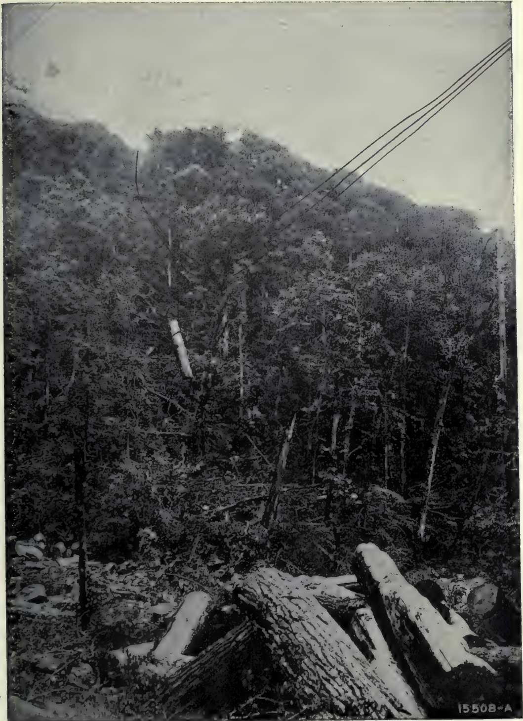
Overhead Skidding, 3000 ft. span, Townsend, Tennessee. (Presented by Messrs. the Clyde, Iron Works Co.)
