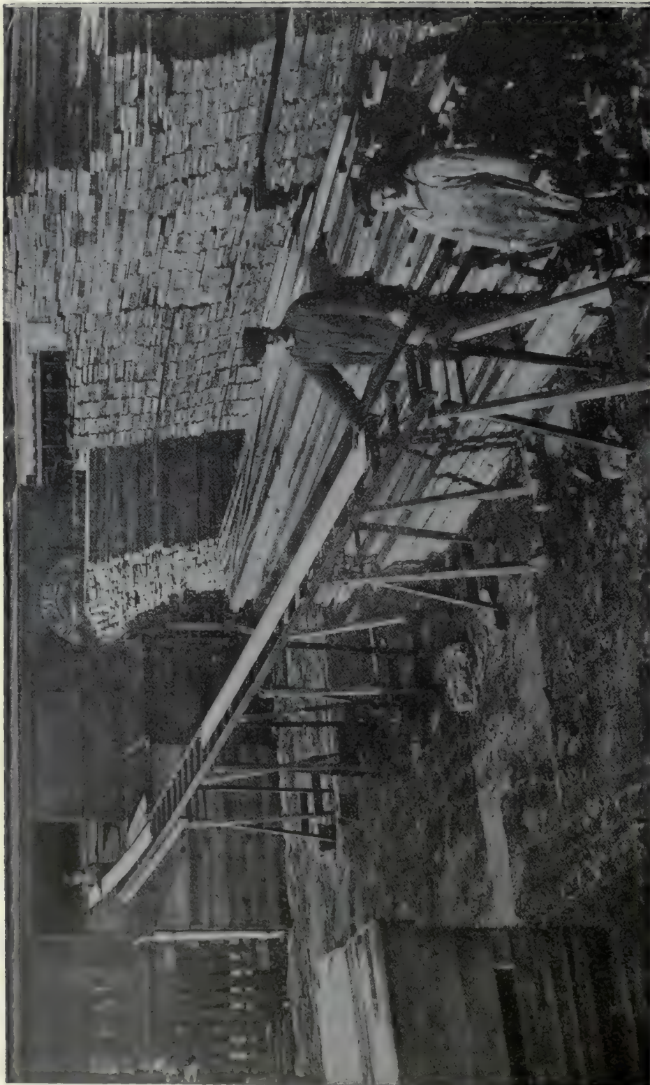
Gravity Conveyor for unloading timber from Railway wagon into yard.
