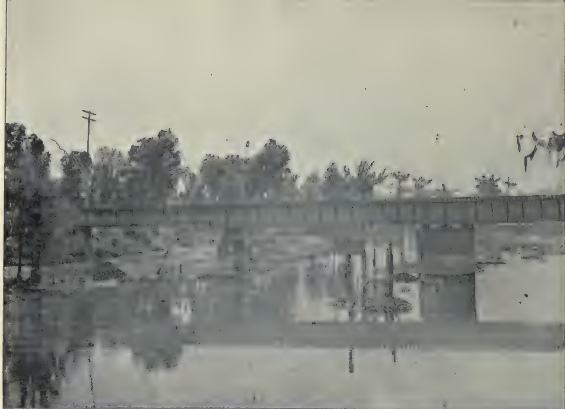
(1). Withlachooshee River, showing flood marks on piers of bridge after the fall of the water level due to the bursting of the dam in February 1918.—Dunellon, Florida.
