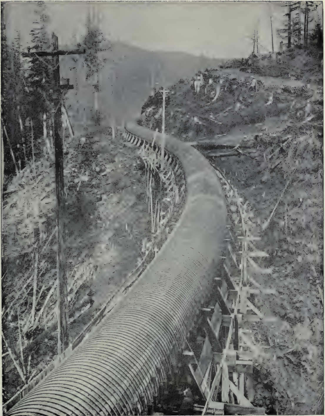
Wood Pipe of Douglas Fir, 6 ft. in diameter, 4 miles long, head 300 ft. delivering water to a power plant in British Columbia. (Presented by B. C. Forest Service).
