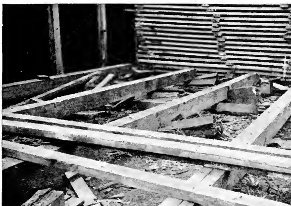
FIG. 140.—A Lumber Pile Foundation which has been poorly constructed and the Surroundings of which are in an Insanitary Condition.
