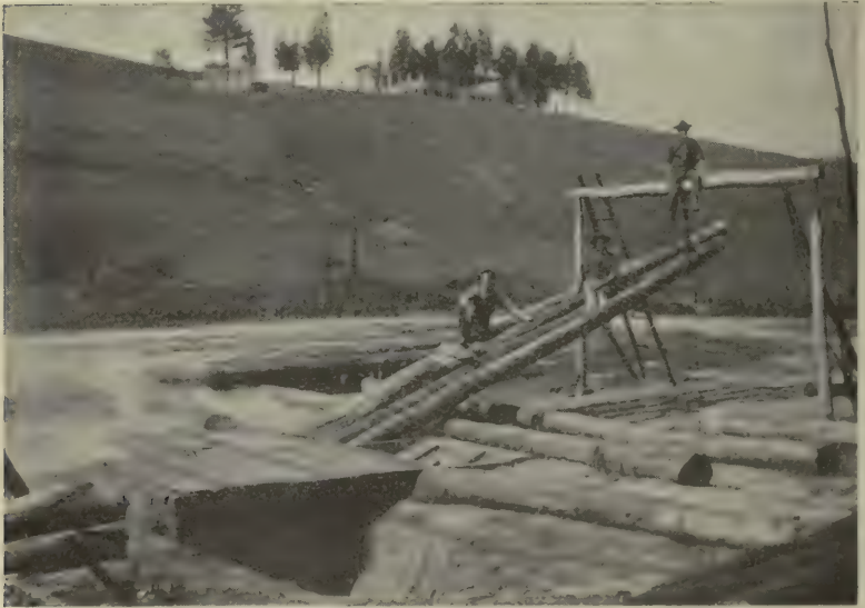
Open-Tank Method of Creosote Treatment Here applied to butts of chestnut poles
