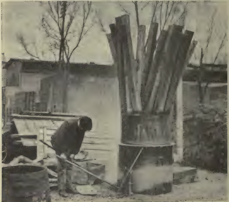
Simple Method of Treating Butts of Fence-Posts with Creosote Plate 25—Lumber and Its Uses
