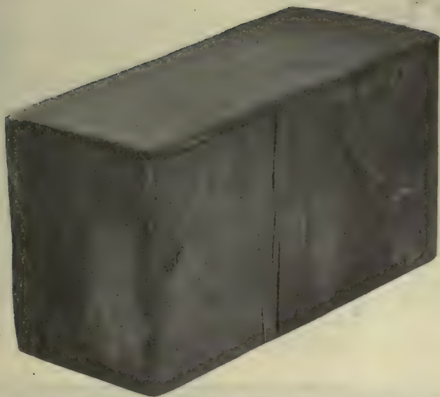
Creosoted Block of Longleaf Pine after Five Years' Service in Congress Street Pavement, Chicago, Ill.
