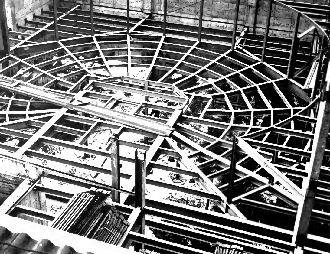
ARTISTRY IN STEEL —The structural framework for the arena theatre provides an interesting study in symmetry. Part of the new Academic Center, the theatre will have a thrust-type stage and a seating capacity of 219.
