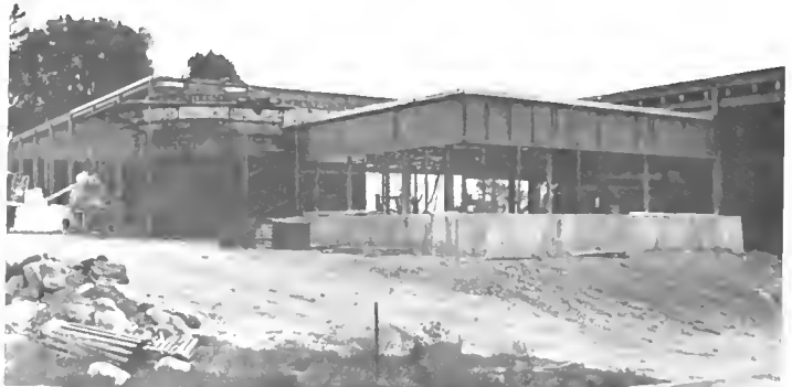
BLUEPRINT TRANSFORMED —What seven months ago was little more than some lines on paper—the new Physical Education and Recreation Center—is gradually turning into the real thing. Since this photo was taken, crews have almost completely enclosed the building supporting the roof and have laid about two complete walls of bricks. By Thanksgiving, most of the exterior work should be completed.
