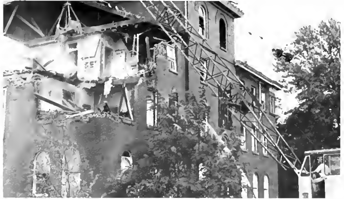
Wrecking crews took apart ancient Bradley Hall piece by piece in mid-August. Work moved quickly but cautiously because of the old building's proximity to the Science Building.
