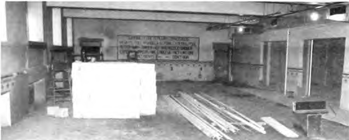
Swiftly and surely, old Hilltop Gymnasium is being converted into Lycoming's new arts complex. Above left, workers for Lindy Construction Company, of Williamsport, have erected a huge mechanical shaft on what was the former basketball court, and have carved up the floor into separate rooms and studios with metal studs. Above right, the loading dock and elevator shaft on the north side of the structure is almost complete; it includes an entrance from the quadrangle. In lower photo, the old swimming pool has been filled in with gravel and clay for the sculpture foundry. Note the familiar sign still visible on the rear wall.
