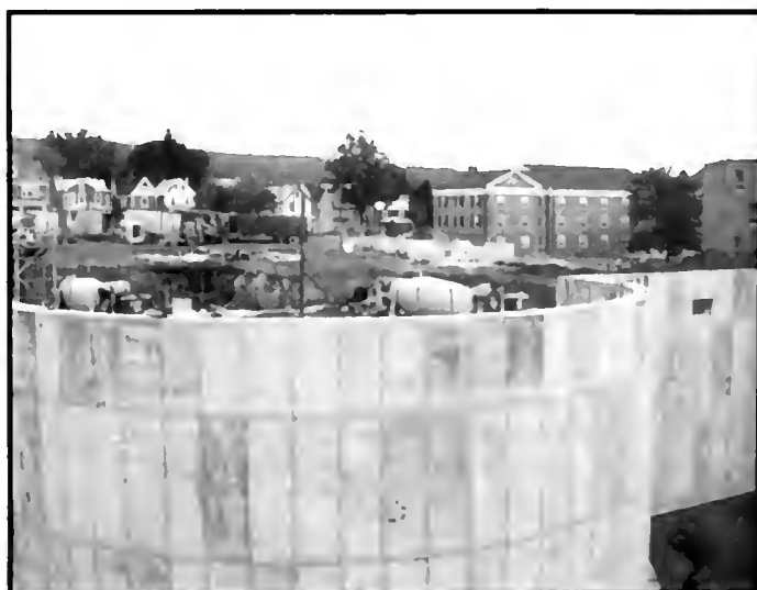
Work on a state-of-the-art science building at Lycoming is proceeding right on schedule. The multi-level building, which will contain a greenhouse, biology and chemistry laboratories, classrooms and offices, is expected to be completed in early 1990
