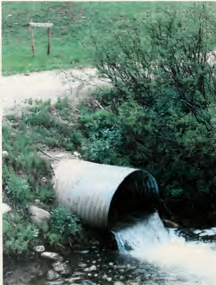
Figure 1. Barrier culvert on FR 9628, upper West Fork Madison River, July 2009.
