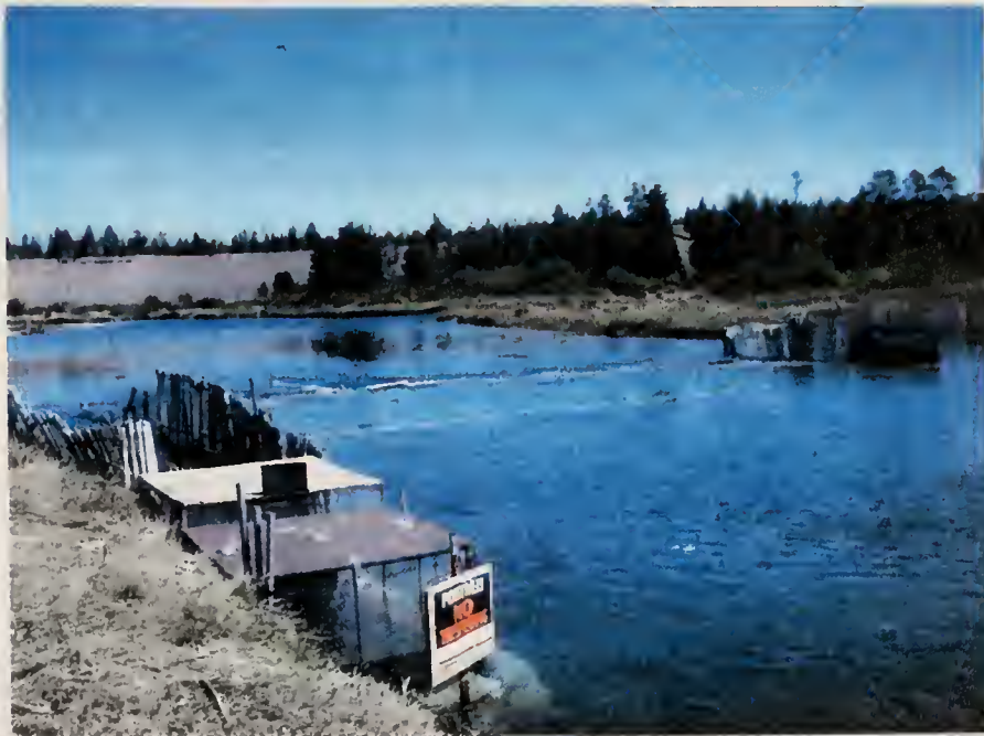
Figure 26. Rigid panel weir used on the Madison River in 2008. MFWP photo by Travis Lohrenz.
