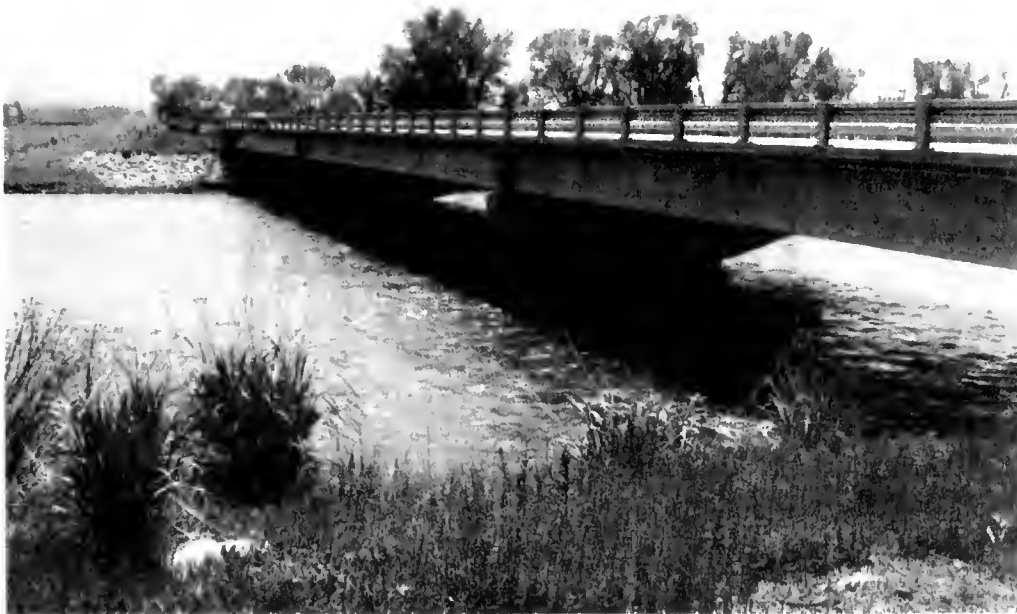
Figure 29. The Madison River at the U.S. Highway 287 Bridge at Ennis, illustrating ice-gorged and ice-free conditions.
