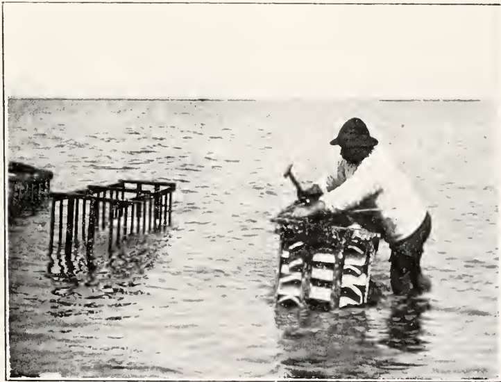
FIG. 13.—NAILING ON THE LAST BATTENS. A RÛCHE FILLED WITH TILES AND COVERED WITH A LAYER OF BRUSHWOOD.
