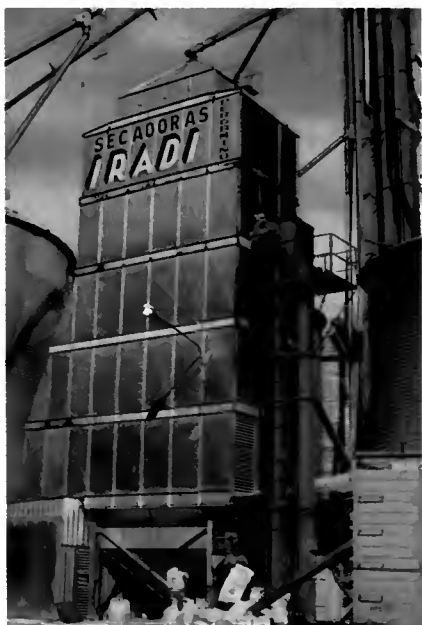
Most country elevators use oil-fired dryers to lower the moisture level in freshly harvested maize.
