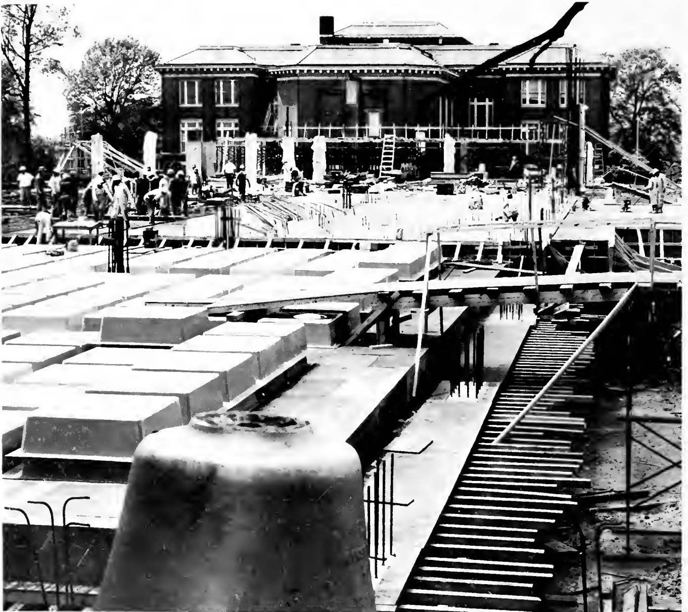
The college campus changes its face in many ways. Workers make preparations for the final pour of concrete on the first floor of the new three-story academic complex. The project is scheduled for completion by the fall semester of 1970.
