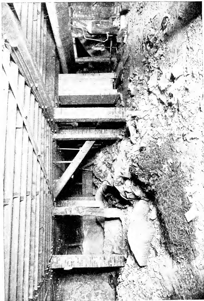
ILLUSTRATION 43. THIS BASEMENT IN THE MAPLEWOOD BAPTIST CHURCH PRESENTS MANY FIRE HAZARDS WHICH SHOULD NOT BE TOLERATED IN ANY PUBLIC BUILDING
